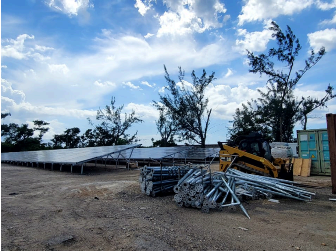
BESS Location Ground Mount Solar System - 330kW Capacity
